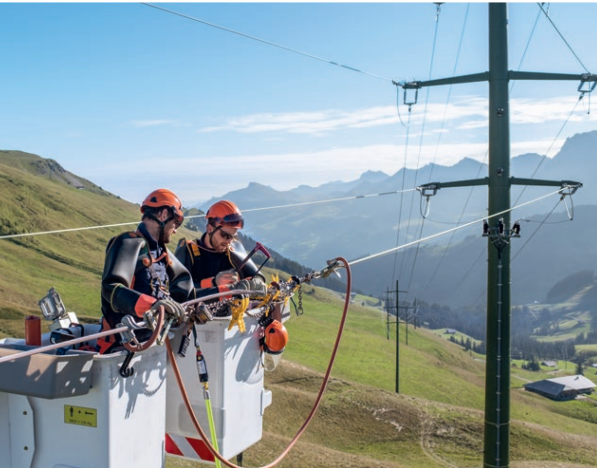
Two grid electricians working on a power line on the Hahnenmoos Pass near Adelboden.
