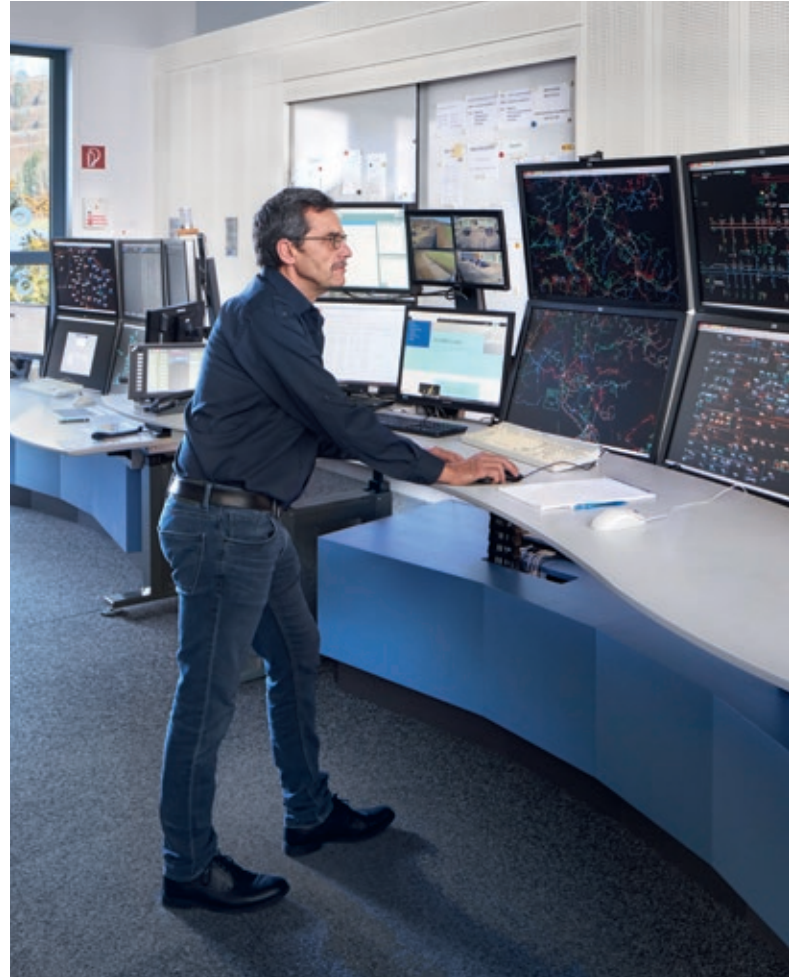
An employee at the Mühleberg Control Center monitors BKW's distribution grid on several monitors.
