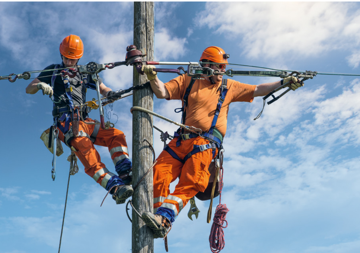
Occupational safety is the top priority. Two grid electricians from BKW Power Grid in action.
