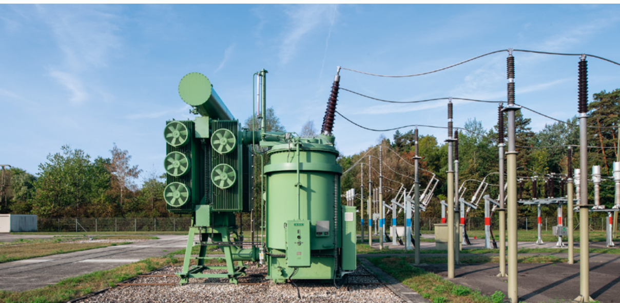
At BKW, transformers are reused whenever possible.
