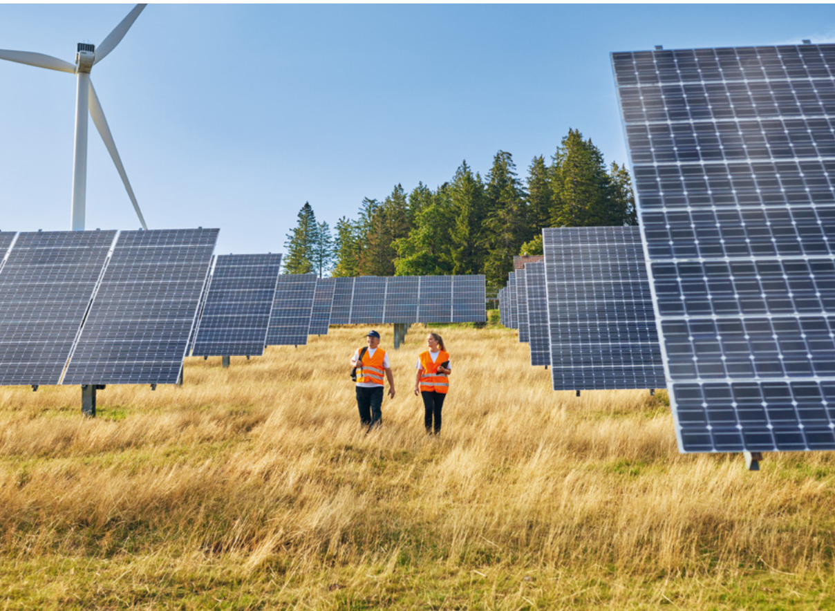
BKW employees check the PV system of the Mont-Soleil solar power plant.
