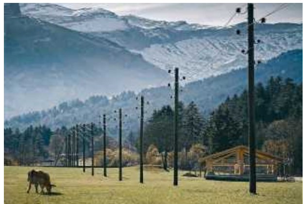
→ The local distribution grid in particular must become smarter at lower voltage levels.
