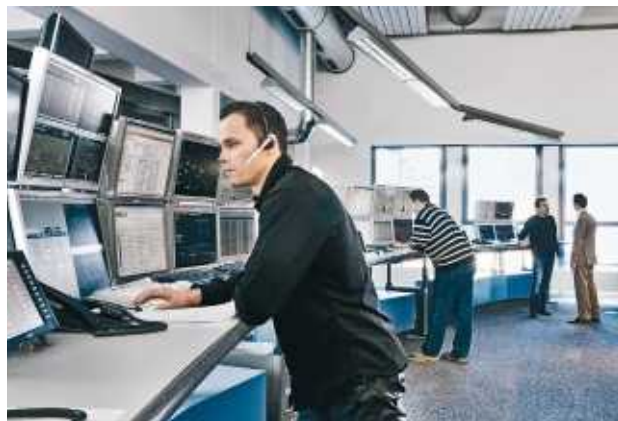
→ The command centre in Mühleberg controls and coordinates the distribution of electricity from the power plants to the regions.
